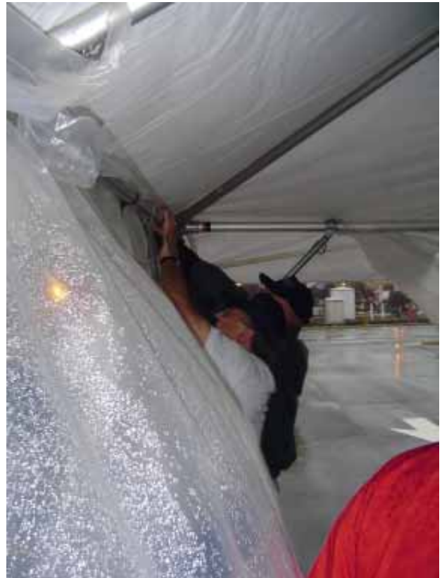
Don & Tim batten down the hatches during rainy gusts. Photos by R. Rodriguez Below: Tim draws the "short" straw and does the electrical plug in!!!
