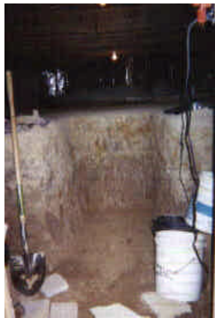
Roy Gurnham's crawl space is seen here during the early excavation stage.
